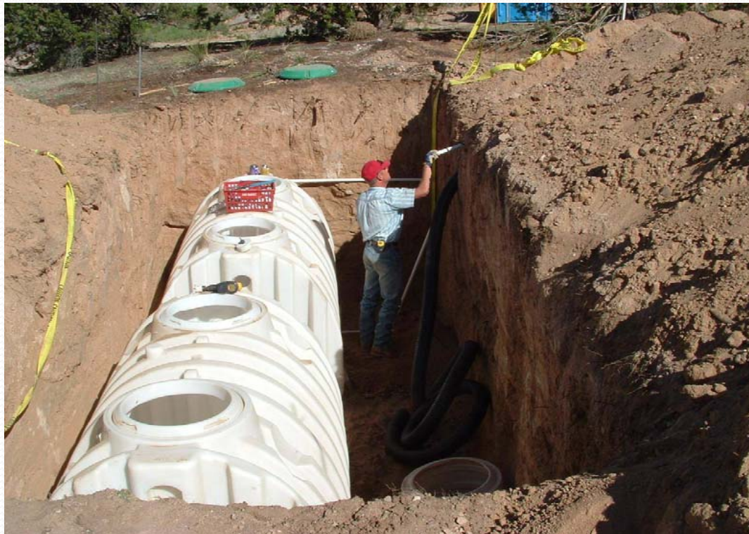
Underground Residential Cistern
